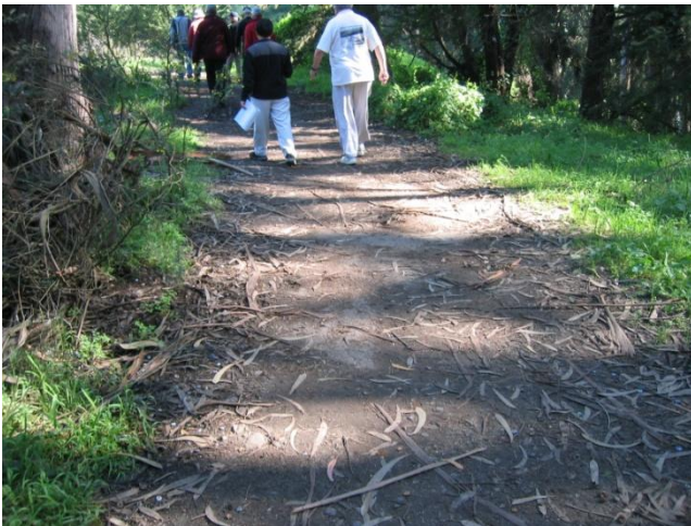
Portion of old roadway between Barnard and Arguello (now a hiking path)
