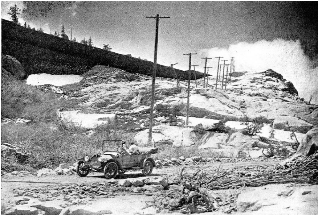
Where the new cut crosses under the Southern Pacific Railroad at the Summit
