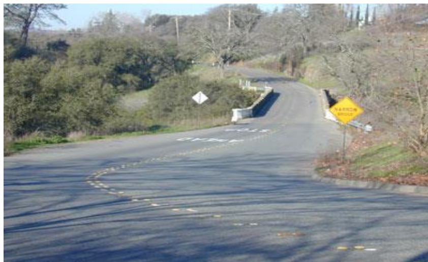
Photo showing erratic approaches and narrow decking of bridge
