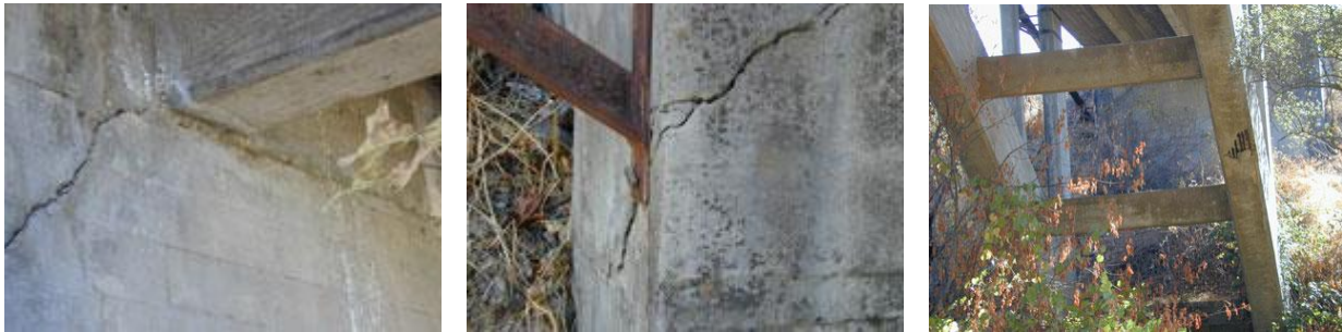
Structural cracks and spalding of rebar requiring need for restoration
